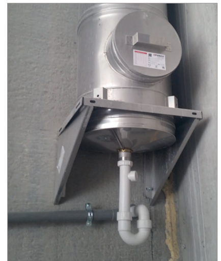
Inspection hatch incl. condensate drainage
